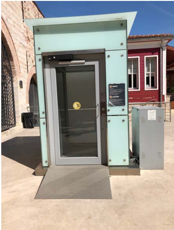
Figure 3.8. Platform lift to the first floor
